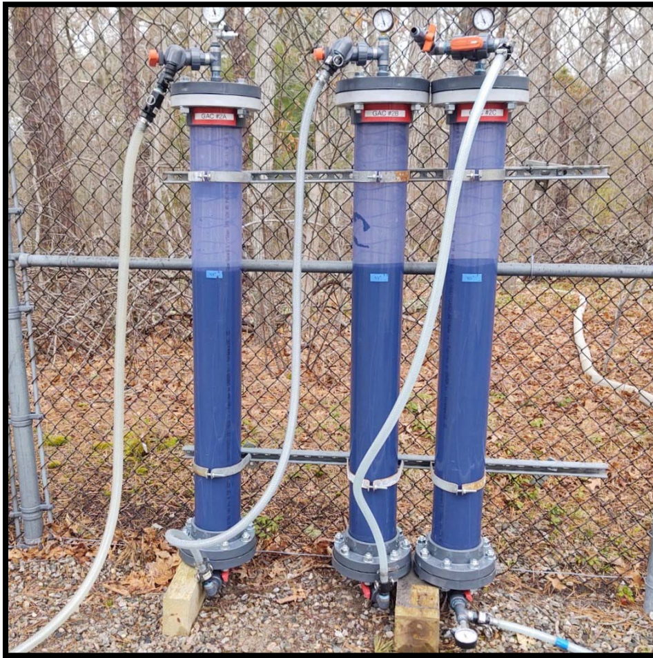
Figure 2.17: GAC Contactor at Hyannisport Station
