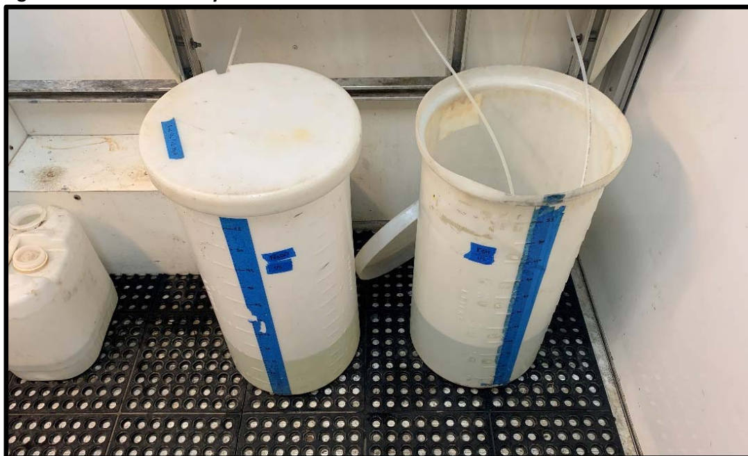
Figure 2.23: Chemical Day Tanks
