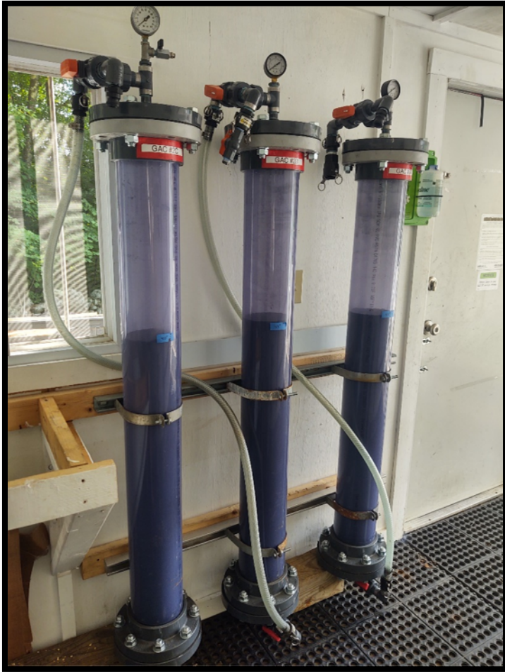
Figure 2.18: GAC Contactors Setup Inside Shipping Container
