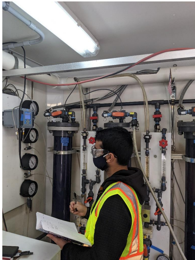
Figure 7-1: Engineer Recording Raw Water Quality Results
