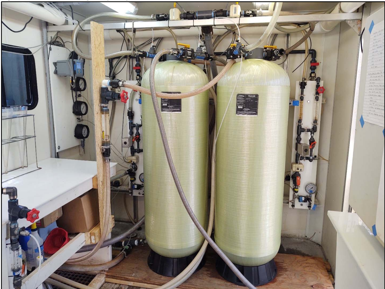
Figure 2.12: 21-inch High-Capacity Greensand Filters
