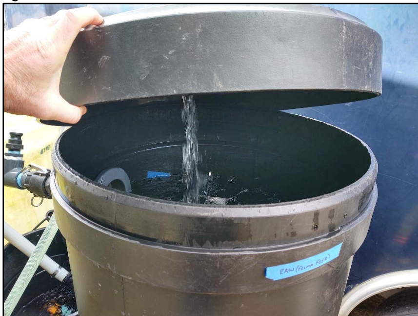
Figure 2.03: Raw Water Break Tank
