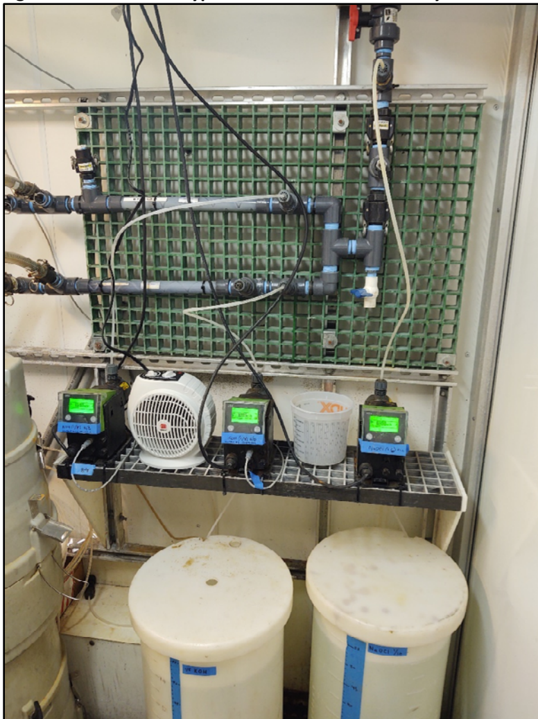
Figure 2.08: Sodium Hypochlorite and Potassium Hydroxide Feed Pumps
