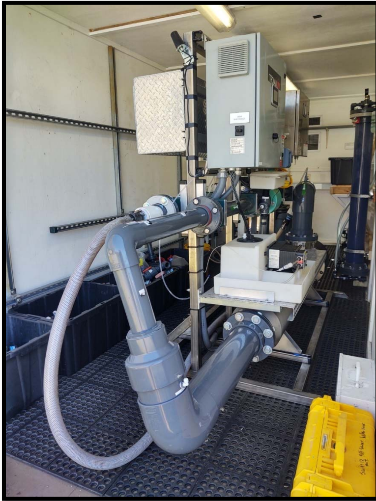
Figure 2.14: UV Pilot Skid Installed in Shipping Container
