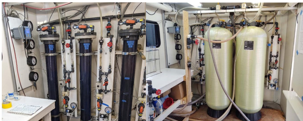
Figure 4-1: Initial Testing Greensand Filters (left), High-Capacity Greensand Filters (right)
