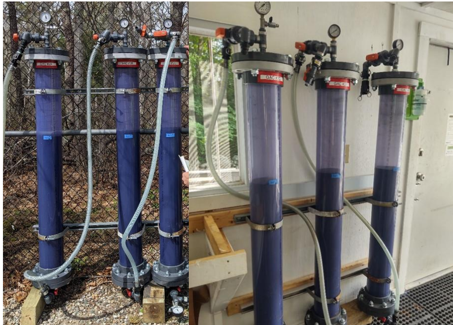
Figure 6-1: GAC Contactors for Initial Testing (left), GAC Contactors Downstream of UV-AOP (right)
