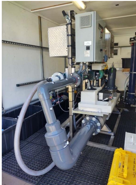
Figure 5-1: Trojan UV Phox 12AL30 UV-Oxidation System Being Piloted
